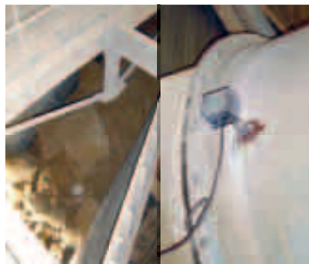
Crusher plant filter protected by an advanced Electrodynamic unit
