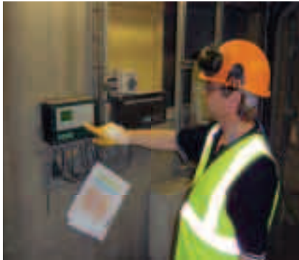
Filter condition assessed remotely
