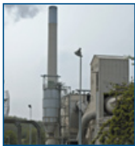
A Cement Kiln Baghouse incorporating an Electrodynamic filter management system
