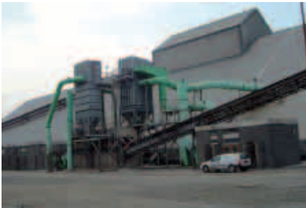
Bag filters found on Electrolytic reduction and smelting processes utilise networked DT990 systems
