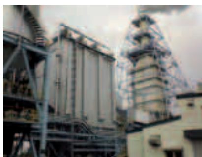
Dynamic Opacity monitor used to monitor electro-filter after calciner
