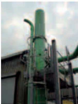
Bag filter performance monitoring of casting bag filter
