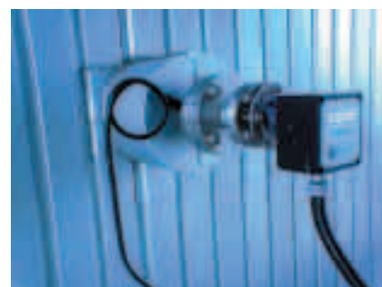
Dynamic Opacity monitor approved to TUV / MCERTS fitted to an electro-filter stack
