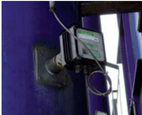
Emissions at hot rolling line monitored by PCME Electrodynamic® System
