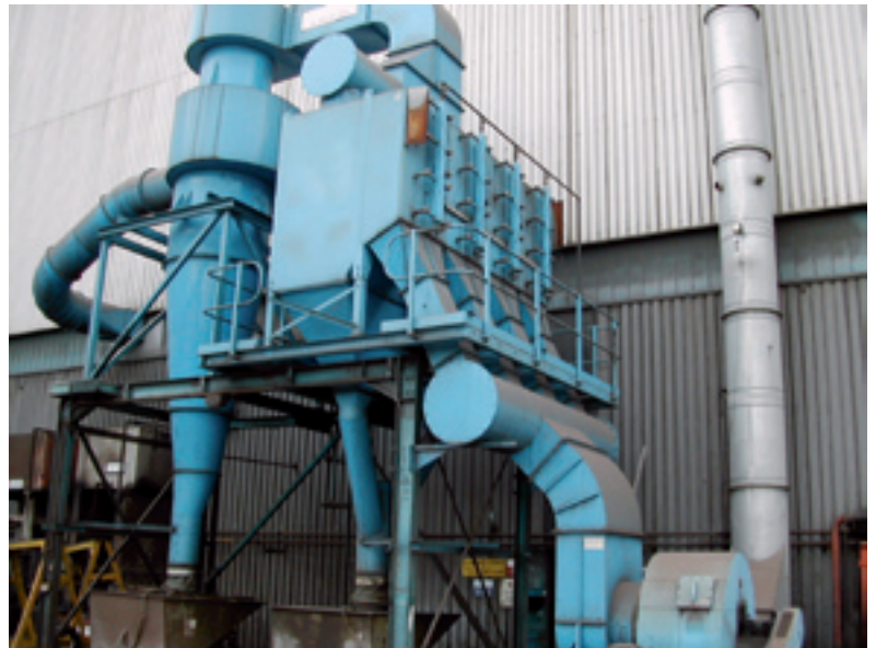
Cartridge filters fitted on rolling mills at stainless steel plant
