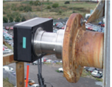
Gas Fired Boiler monitored by Pro-Scatter Technology
