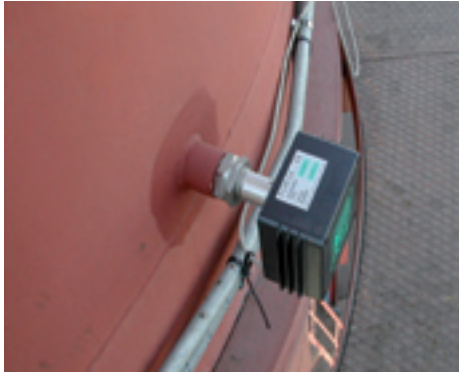
Electrodynamic Instrument monitoring stack on primary extraction system for Electric Arc Furnace
