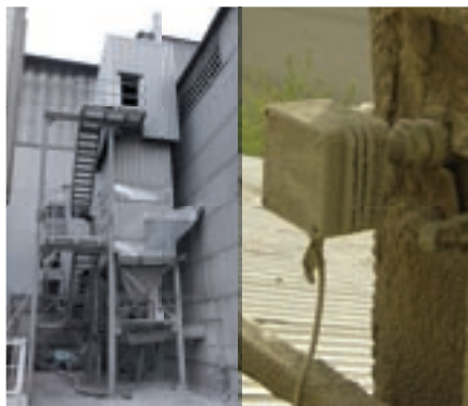
Damp cement mill monitored utilising a fully insulated sensor
