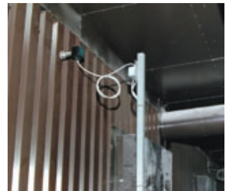
Filter chamber performance continuously monitored via a networked Electrodynamic system
