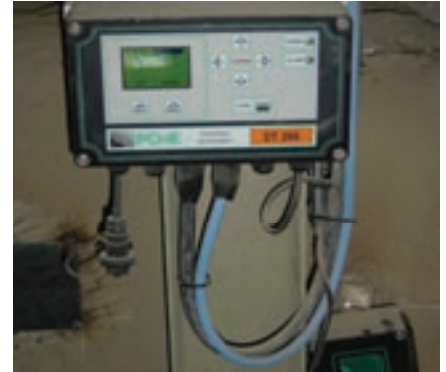
Product loss prevented by silo monitoring
